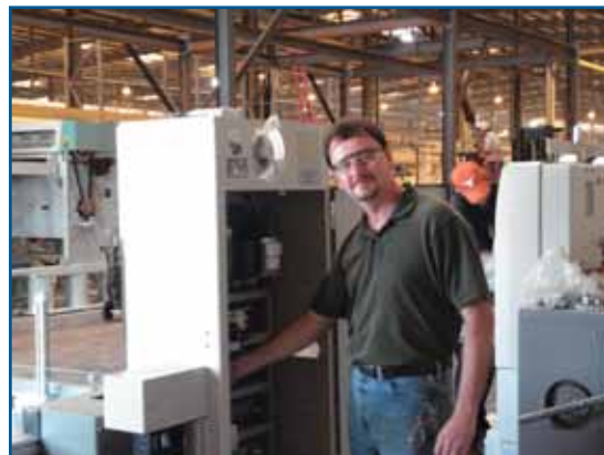
John Morris, Area Engineer for BOPP, checking the configuration of an electrical panel.
